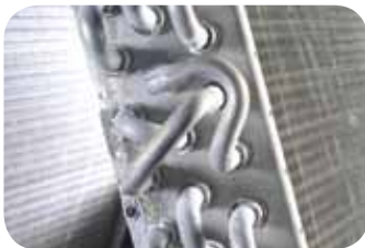
Aluminum tube and tube sheet after 500 hours in a controlled corrosive environment.
